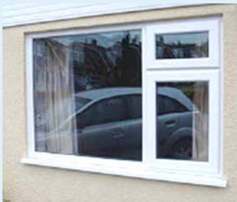
Inappropriate UPVC Window
