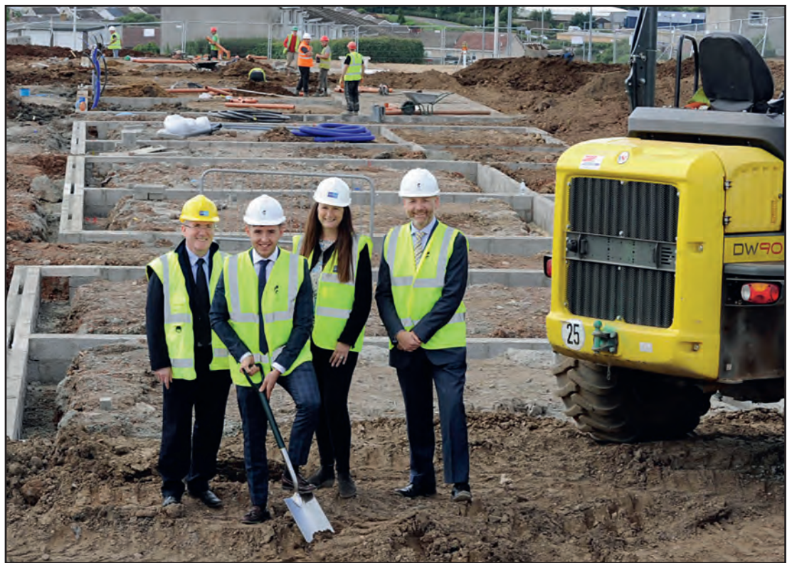
WORK BEGINS: SLC’s Daniel Lowe, Councillor Josh Wilson, SLC’s Annette Finnan and Bruce Lindsay, Development Manager at CCG at Belstane Gate
